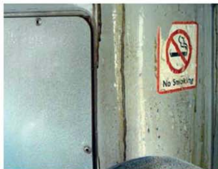
The lower deck GRP has bubbled, but is intact
